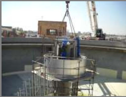
Figure 2 : Northern Wastewater Treatment Works: Raw Sludge Thickeners completion of central pivot to support new bridge.
